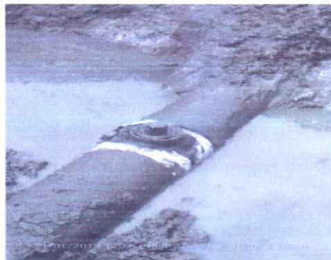
SPILL POINT AFTER EXCAVATION
